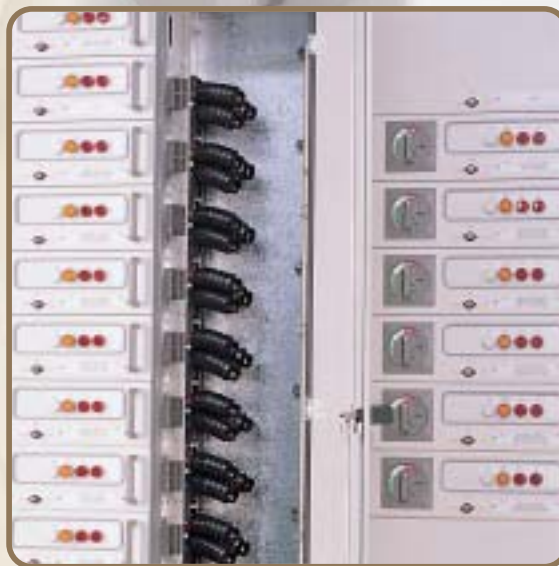
View into the cable compartment
